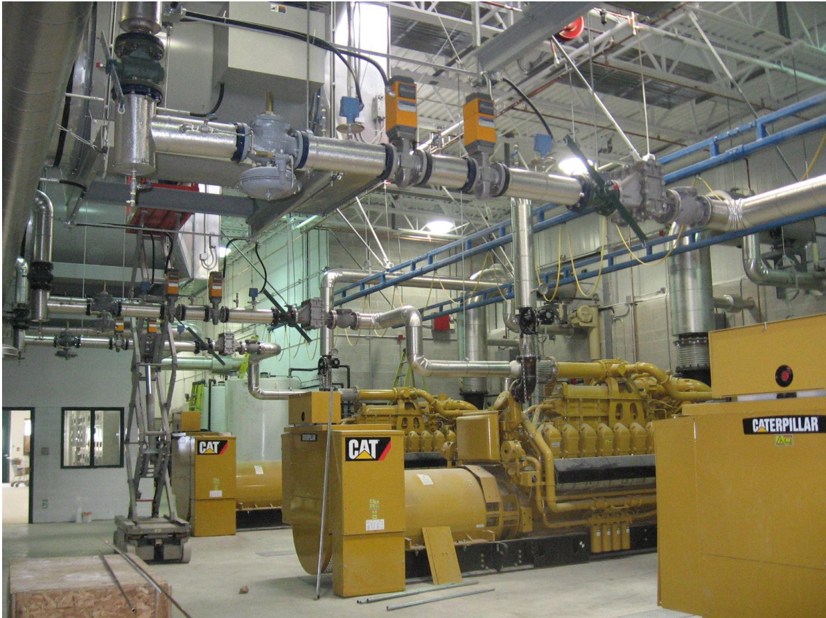
Landfill Gas to Energy Plant Engines
