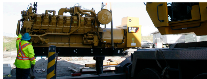
One of five engines arriving at the facility, which will convert landfill gas to electricity.
